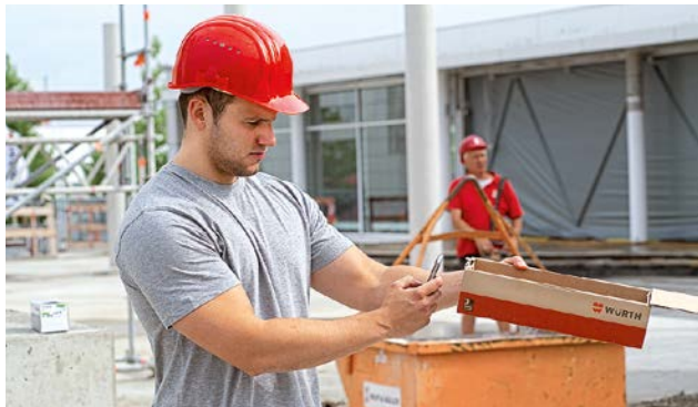
Our customers can use the Würth App to order products directly at the construction site.
